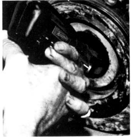
Surface treatment is applied to bearing housing by means of a "gun" holding the electrode material.
